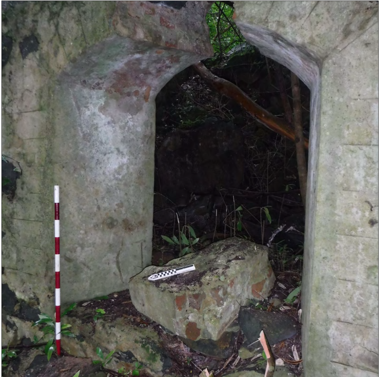
Figure 36. Interior view of doorway to pump house structure (Feature 1 at Site 5), view west; note, north arrow is in error by 180 degrees (north is to the right in this view)
