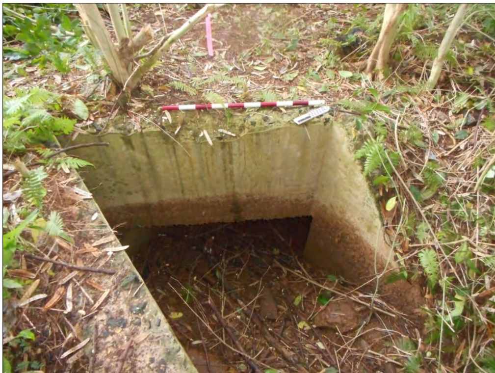
Figure 12. Another view of Feature 1 (Site 1), facing northwest; rectangular-shaped culvert below the photo scale goes under the road leading to the airstrip.
