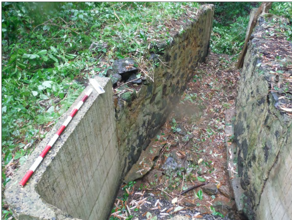
Figure 20. Another view of Feature 3 (Site 1), facing north; note use of varied materials and methods (poured-in-place concrete as well as shaped basalt boulders and mortar).
