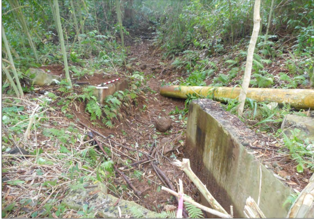
Figure 11. Overview of Feature 1 (Site 1) (concrete sluice-gate and culvert), view south; earthen ditch extends out of the image to the south; note, displaced water pipe to the right.
